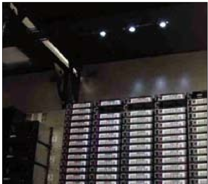
IBM TS3500 - LED lighting
