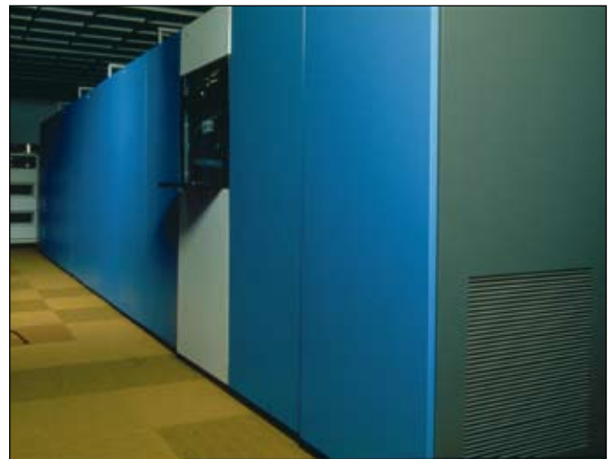
IBM MSS 3850 in the data center in the background on the right
