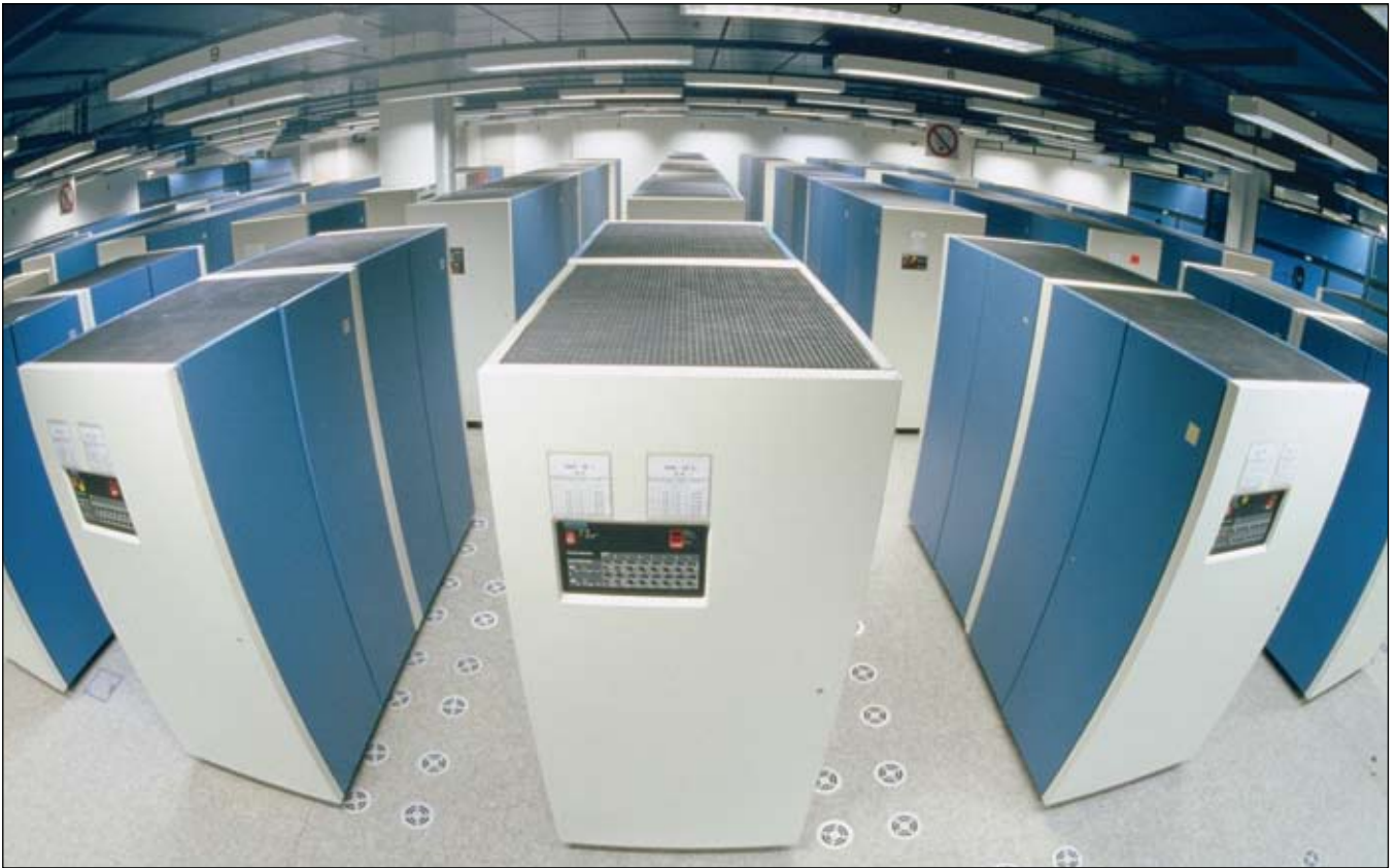
At that time, IBM 3380 disks and 3880 control units filled entire data center halls
